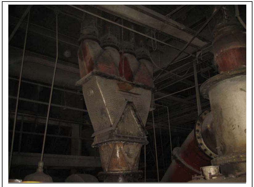
Figure 2 Boiler Fuel Line Riffles Above Coal Pulverizer
